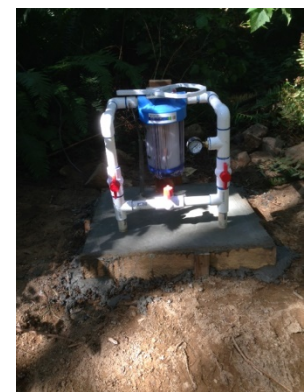
Figure 22: A water filter installed in 2016.
